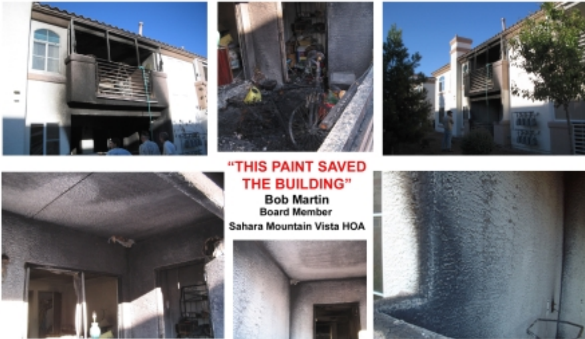
Though the paint is carbonized, the underlying substrate is intact and can be easily rehabilitated.
